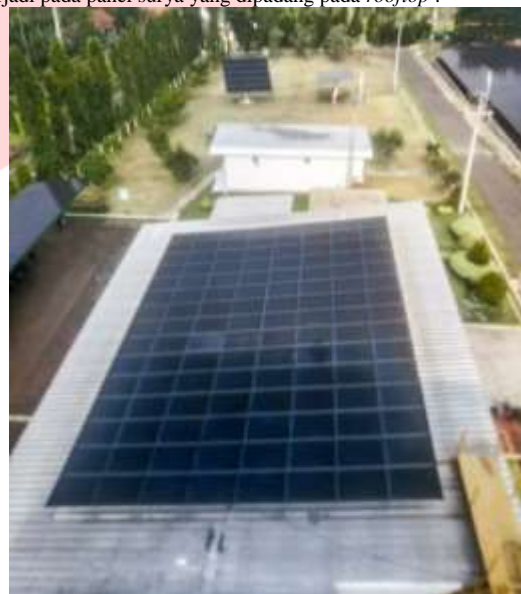
Gambar 4. 7 Rooftop Terkena Shading
