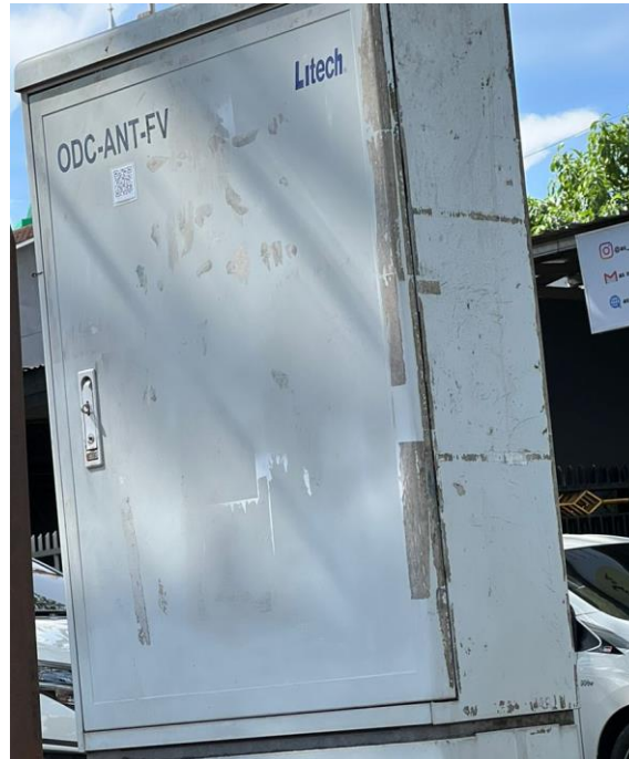
Gambar 2.3 Optical Distribution Cabinet.
