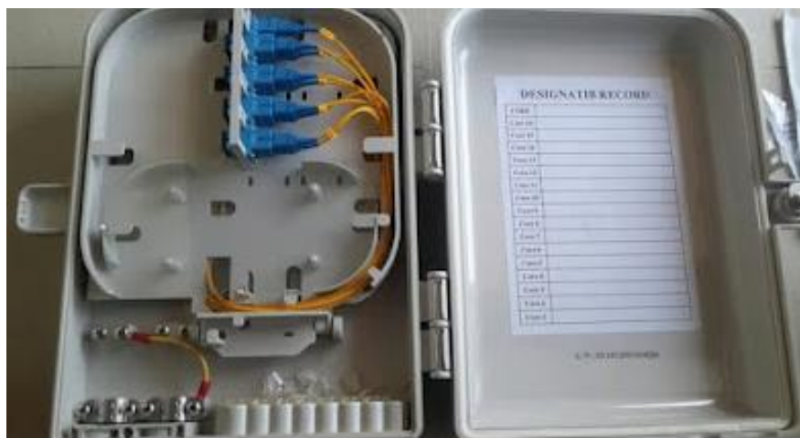
Gambar 2.4 Optical Distribution Point.
