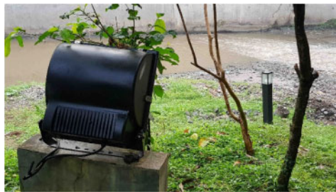
Figure 5. Flood lighting directed to river stream.
