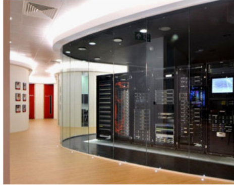
Figure 4. Server room, on-premises data storage. Source: pinterest
